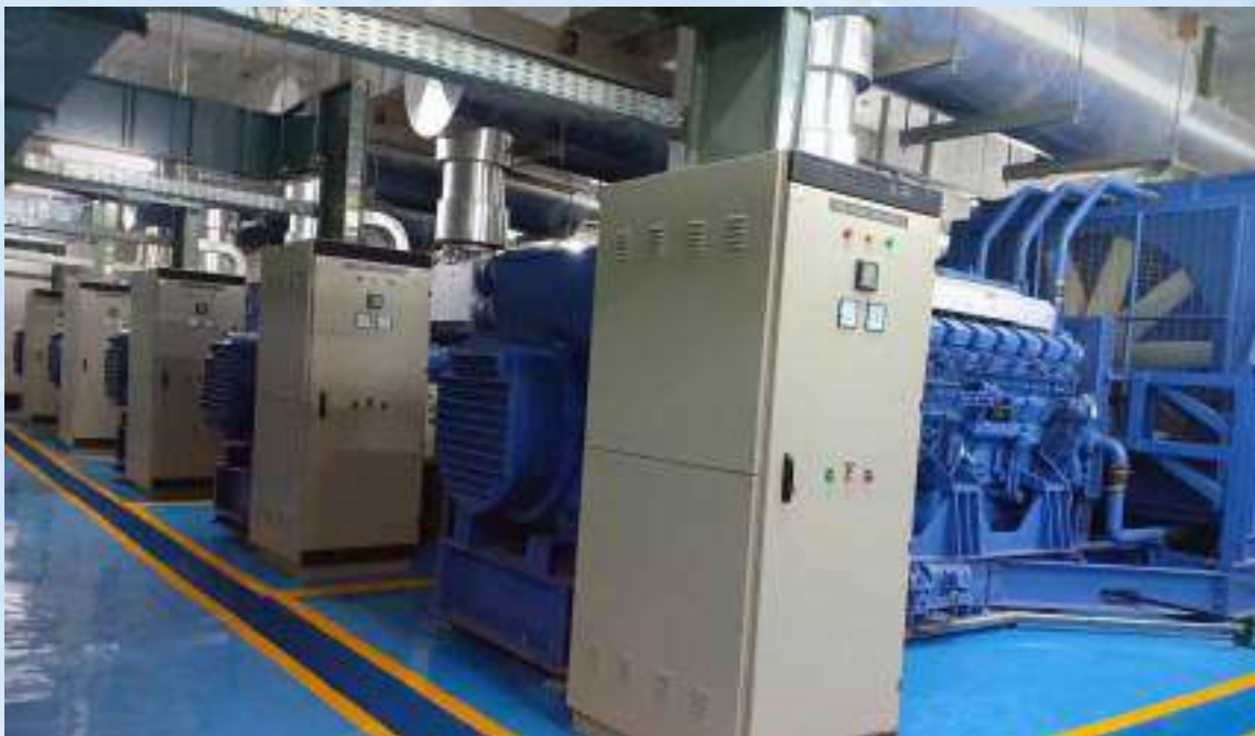
District-8 @ SCBD Senopati, Jakarta 9 x 2015 KVA, 5 x 2250 KVA
