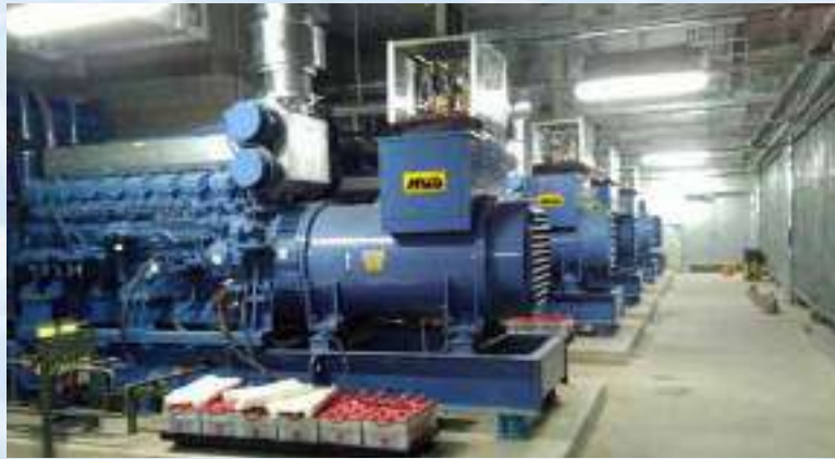
BTPN TOWER - 5 x 2015 KVA
