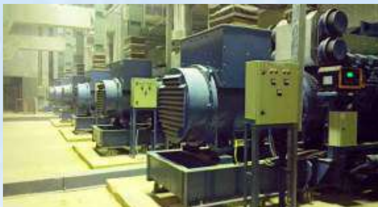
GAMA TOWER - 6 x 2015 KVA
