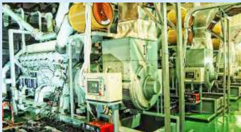
GRAND INDONESIA (I) - 1 x 1920 KVA + 3 x 2020 KVA
